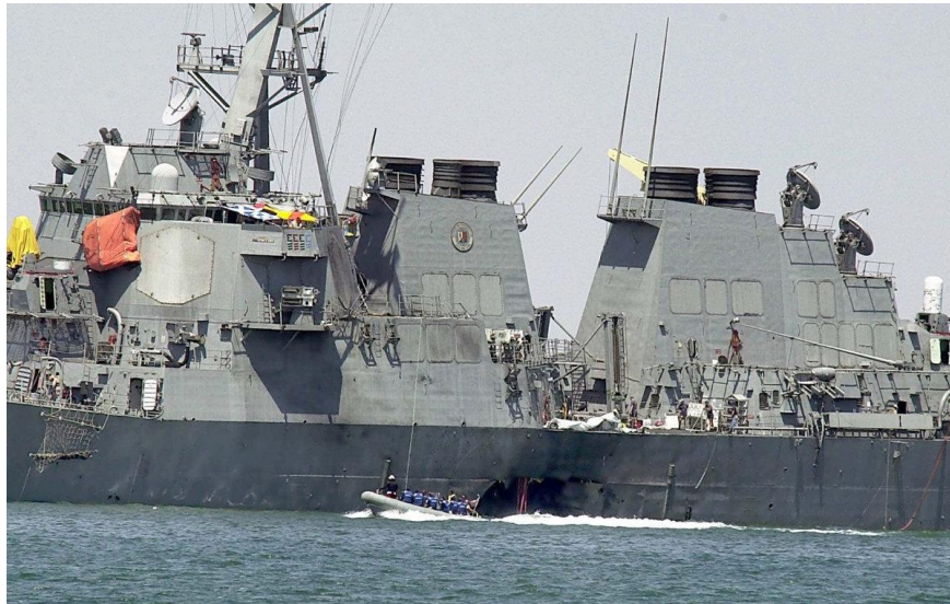
Experts in a speed boat examine the hull of the USS Cole at the Yemeni port of Aden on Oct. 15, 2000. A powerful explosion ripped a hole in the U.S. Navy destroyer in the Yemeni port, killing 17 sailors and injuring some 30 others.
